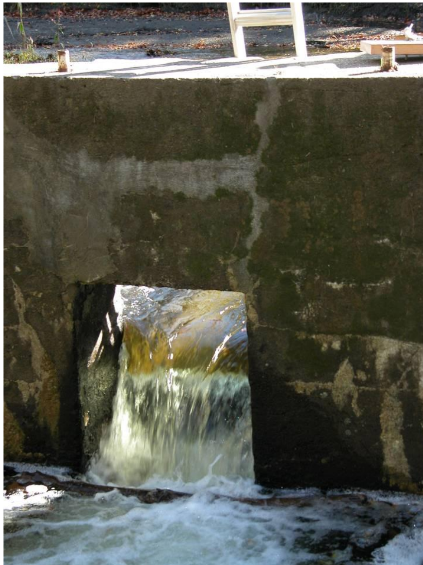
Photograph 6. Downstream face of the dam showing low level outlet with boards removed.
