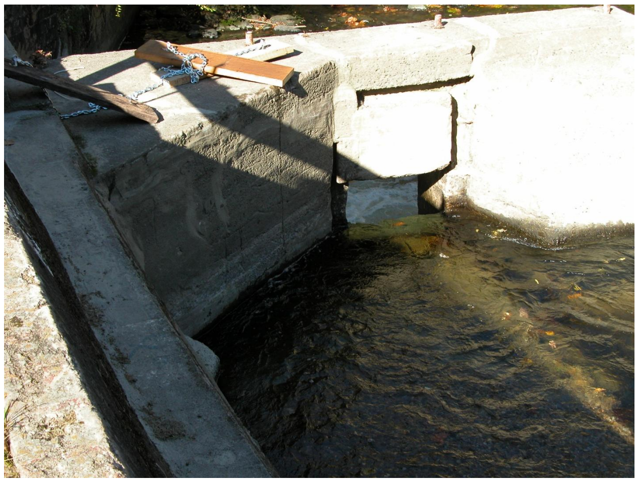
Photograph 5. Upstream face of dam with pond drawn down, showing removable boards and low level outlet.
