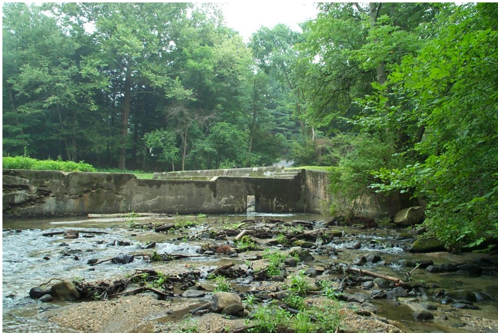
Photograph 2. Old Papermill Pond Dam as seen from downstream with the low level outlet open.
