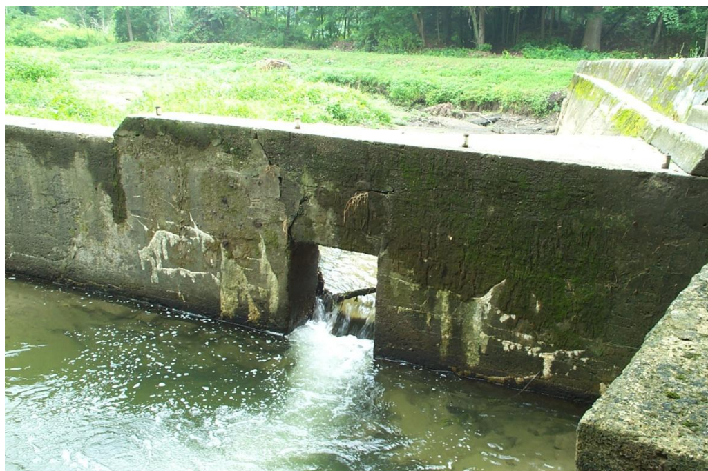
Photograph 3. Old Papermill Pond Dam showing downstream and upstream areas with pond drained.
